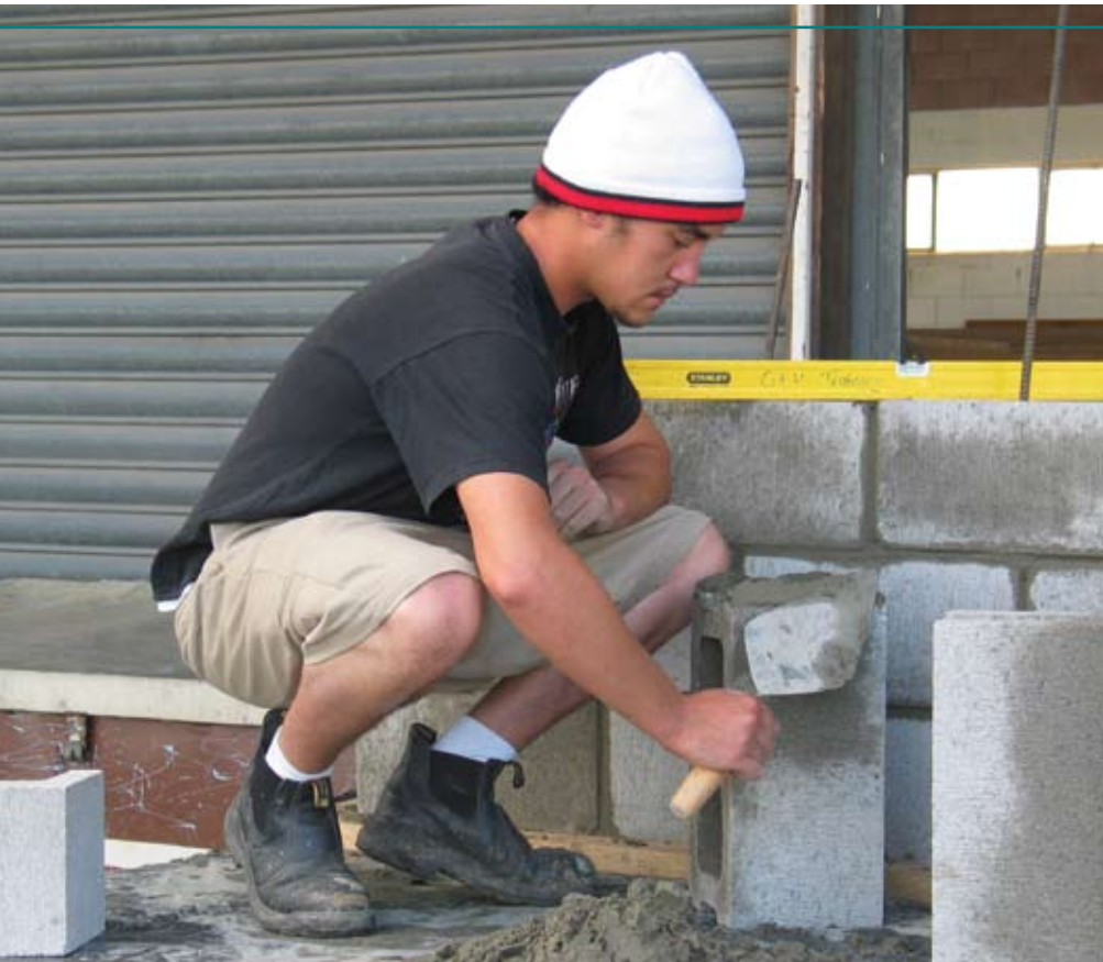
An Industry Partnerships bricklaying programme run in Whangarei, helped trainees like Joseph Broughton learn skills to launch a career in construction.
